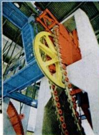
The main drive powers the tram across the river in 3½ minutes.
