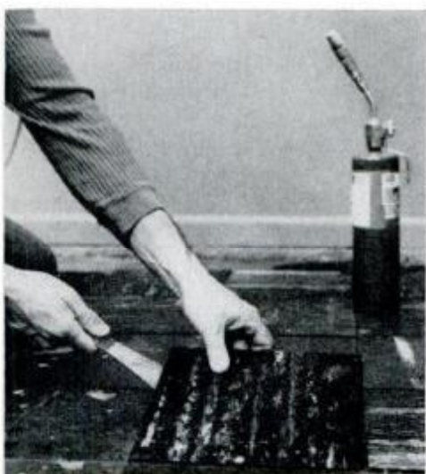
Old tiles are removed from concrete slab with stiff-blade scraper, propane torch.
