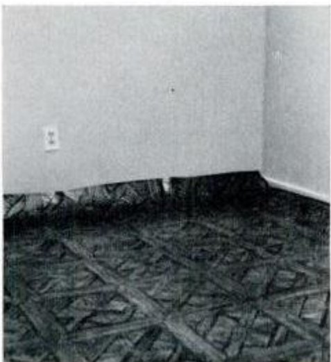
Oversize floor covering is laid to curve up three walls, then is trimmed to size.
