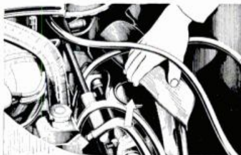
Upper mounts of front shocks are often reached from inside engine compartment.
