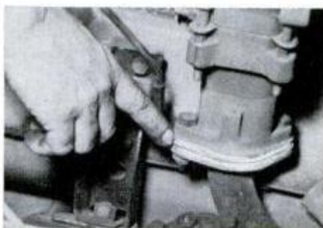
Exhaust manifold and exhaust pipe flange should be checked for leaks.
