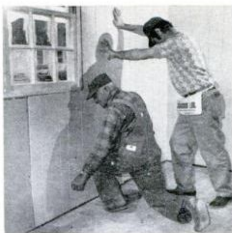
Hold panel in place, bang on face, and hope that an accurate line is transferred.
