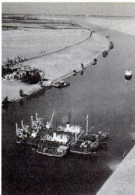
The powerful YHLCs are positioned in the middle of the canal, a section of the concrete caisson cradled between them.
