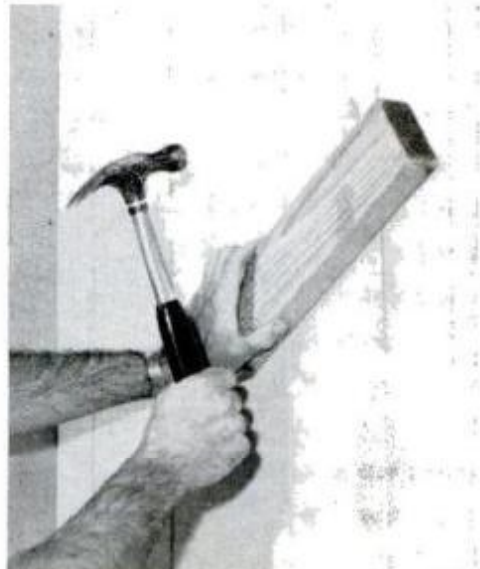
Finally, distribute adhesive evenly by sliding block of hardwood over surface while tapping continuously with hammer.
