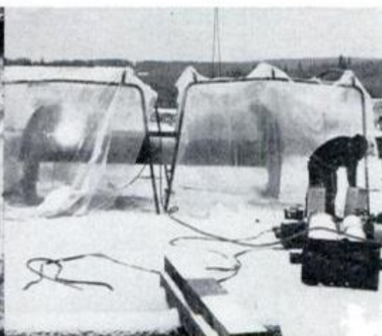
Working under tentlike plastic shelters to protect them from the intense Arctic cold, welders join sections of steel pipe.
