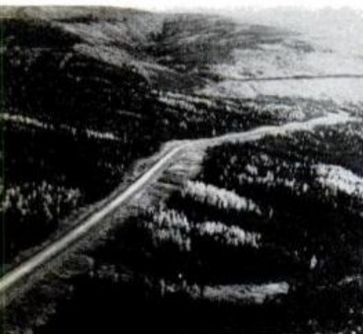
Aerial view shows service road bulldozed through trackless regions of the Arctic to carry machinery to construction sites.
