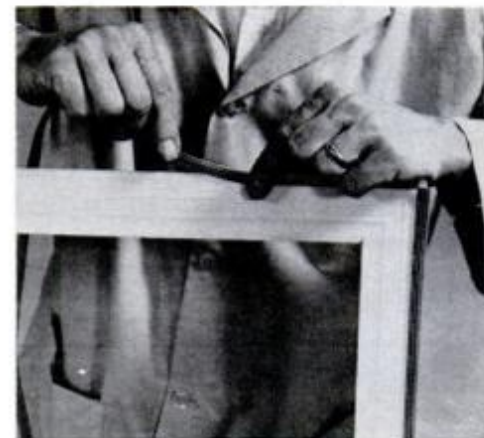
5. Reinstall the original rubber gasket that was taken from the old storm-door glass over edges of new plastic frame.
