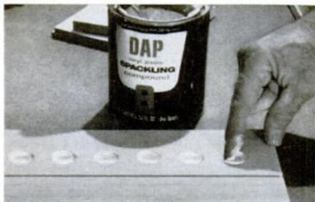
Fill pilot holes with vinyl spackling compound and let dry. Overfill holes a bit to avoid shrinking.
