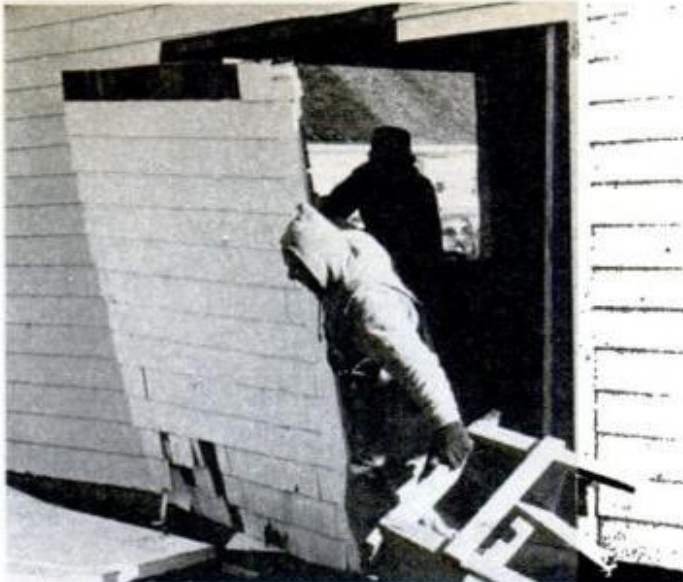
Wall section comes down fast. Because wall was first framed, there is no need for a temporary support wall.
