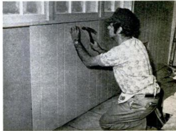
Paneling is secured in place by driving precolored nails that match panel color.
