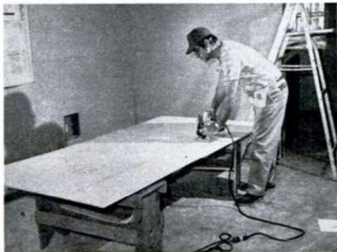
Window cutout in panel is made from back side, using circular saw. To start, use a vertical plunge cut.
