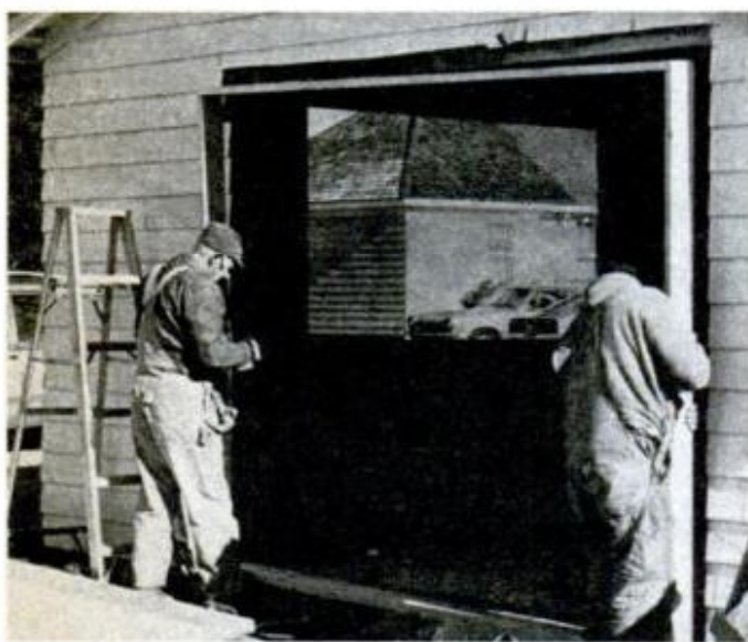
Two men push frame into opening. After plumbing frame with level, it is fastened to studs with screws.
