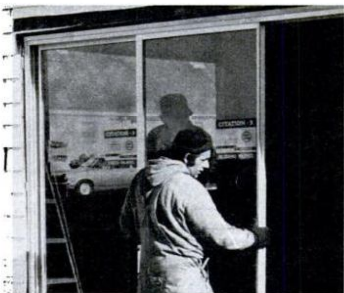
Last step is to install door itself. Door shown is fully weatherstripped to minimize air infiltration.
