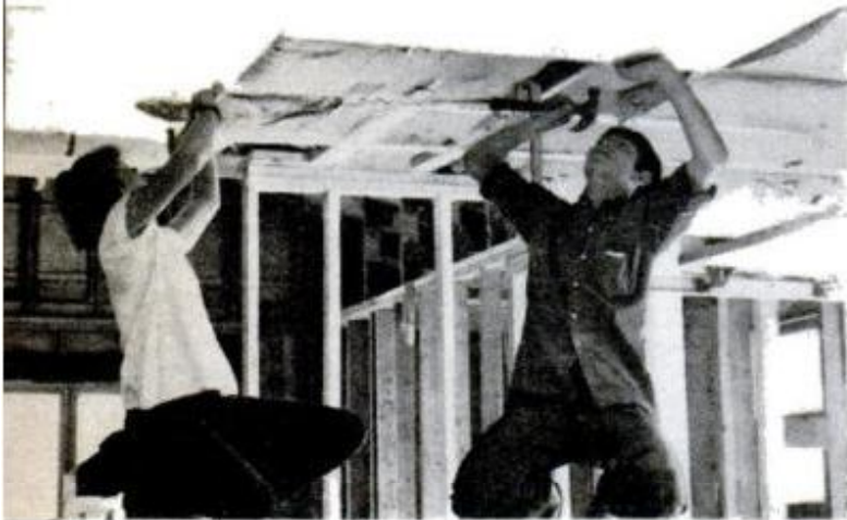
Plasterboard ceiling goes up fast with two energetic youngsters wielding their hammers.
