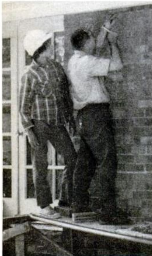
Instructor Watson gives a student pointers on installation of the top course of brick veneer used on house exterior.
