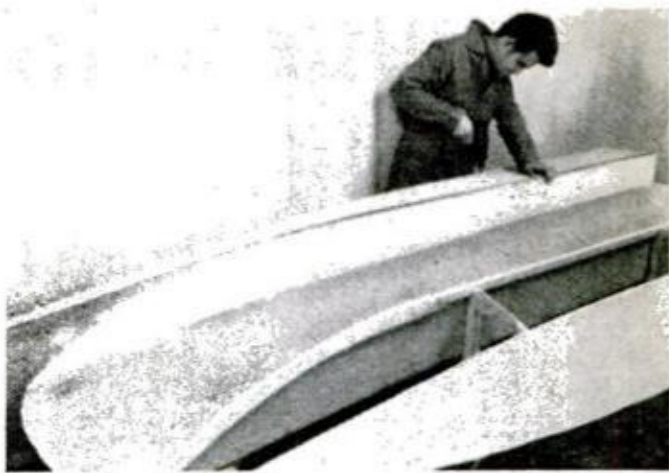
Bottom runner planking is installed in same manner as side planking. Panels will be found to bend easily into place. Fastenings are used along longitudinals.
