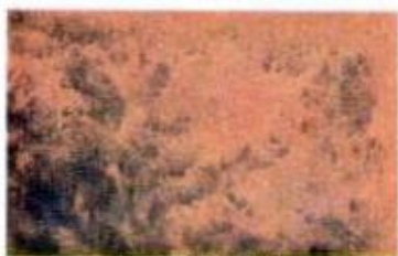
Rusted Metal Before Treatment
