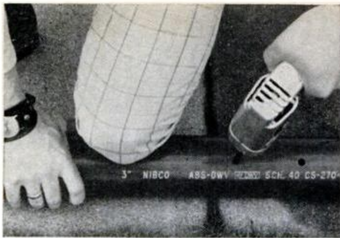
Drill drainage holes, \frac{1}{4} in. in diameter, 4 in. apart in bottom of pipe so remaining water will drain out.
