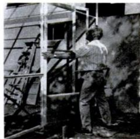
Closure channel is attached to the doorbars and the door is hung in the gable end of the structure.
