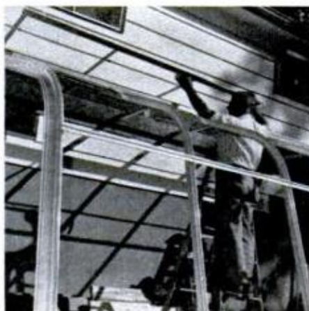
Operable vent sash is next to be installed. Vent operates by thermostat to aid temperature control.
