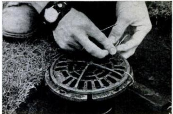
Round grating from a floor drain is attached to closet flange with short lengths of copper wire.
