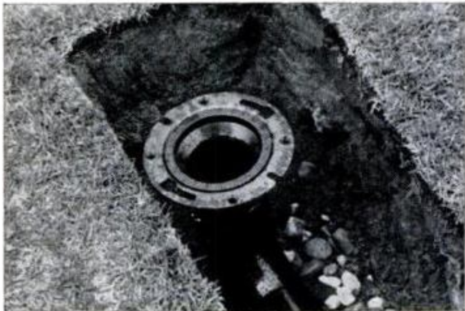
Nibcaware closet flange is attached to far end of drainage pipe to bring grating nearly flush with ground.
