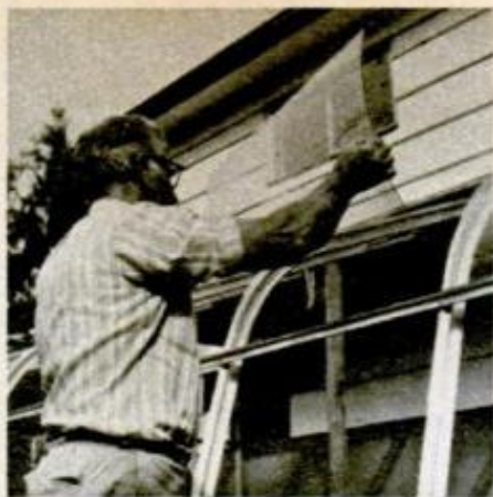
Vent-section glass goes on first, to be followed by panes on the roof, side (above) and gables (ends).
