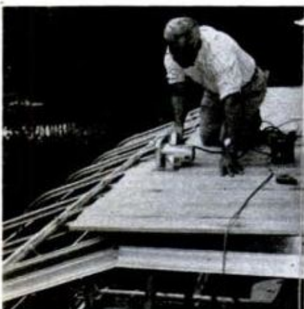
Tongue-and-groove sheathing is fastened to the deck; then, following a chalkline, trimmed in place.
