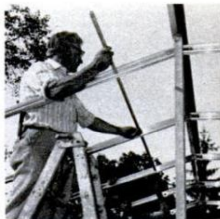
Vent shaft is then positioned and installed after the main members have been fastened in place.
