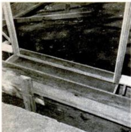
Door frame (jamb) is positioned; the concrete footing—at door center—must be 1 to 2 in. above grade.
