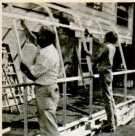
Gauge determines precise location of the eave. Glazing, which follows, locks the structure square.
