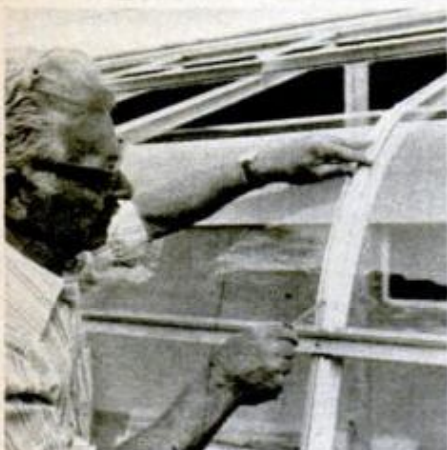
Bar cap is installed immediately, with sheet-metal screws serving to keep the glass pane in place.
