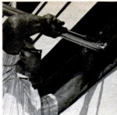
Deck frame is then fastened to the 2x8 header on the house by means of wood screws.
