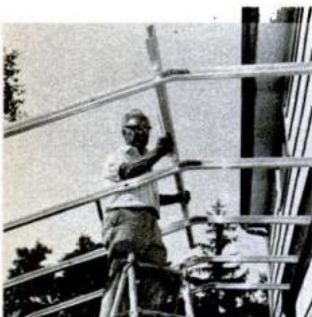
Ridge and 2x4 stringer for deck are attached next. Operable-vent section is located directly below it.
