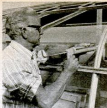
Glass panels are bedded in a foam tape. Joints are then sealed with a top compound similar to caulk.
