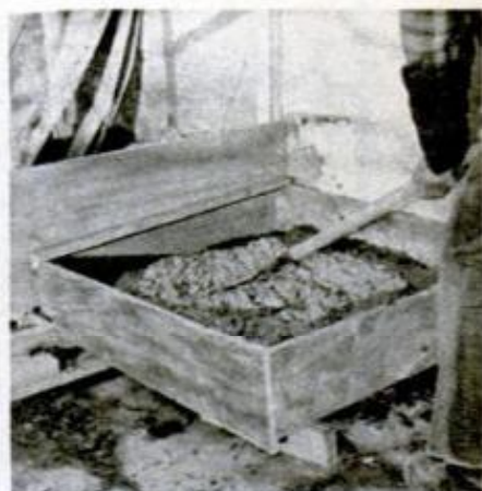
Concrete was pushed into trench through an 8-in.-wide opening in bottom of the pour box.
