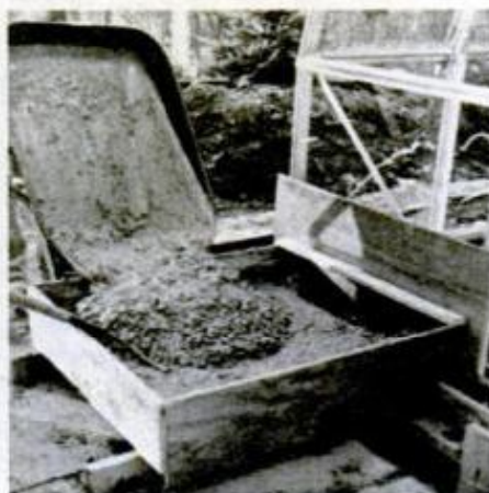
Concrete footings are poured after the frame is up, and glazed, to assure that glass panels will fit.
