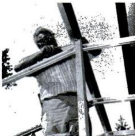
Vertical 2x4s are used temporarily to support the deck stringer during remaining frame assembly.
