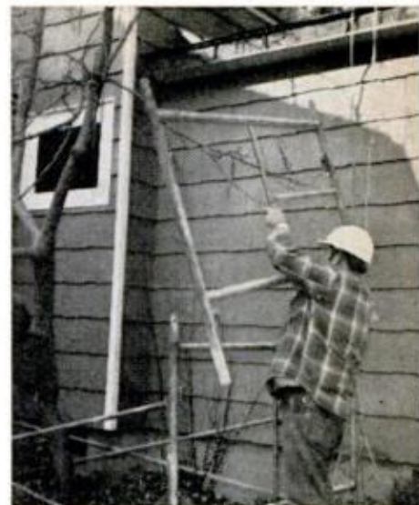
Middle tiers of platforms (center photo) go up simultaneously with end tiers. Right: Second level can be handled easily because man is on the ground.
