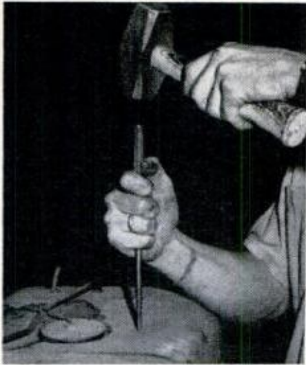
Drain tank, fill it with water and then locate position for Pacemaker.
