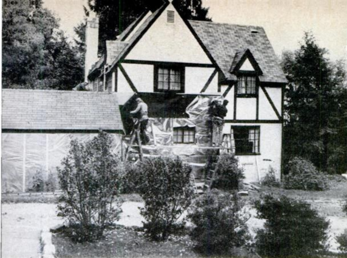
Insulation , felt and aluminum foil went up before the aluminum siding was hung. The insulation used is basically a Styrofoam that comes in large sheets. (A piece of it shows above head of worker on left side of scaffolding.) In lower photo, head mechanic saws siding panel at cutting table.
