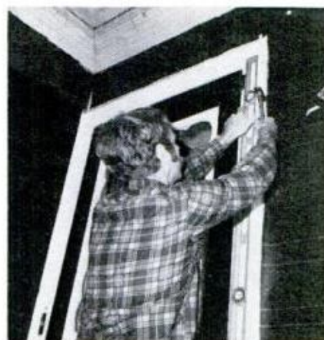
Channel is installed using spirit level. Casing reveal (exposed width) should be the same throughout job.
