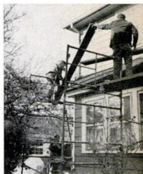
Each pair of braces is connected and pivots at center. Once these are installed (see below) scaffolding is rigid, planking can go up (photo right).
