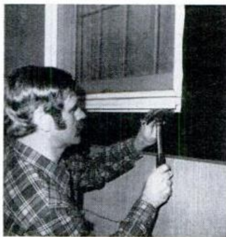
J-channel is nailed to underside of sill; sill ends are notched to suit vertical channels which go up next.
