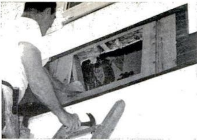
Siding (asbestos shingles, here) is removed, sheathing is cut away. If stud is in opening, it too is cut out.
