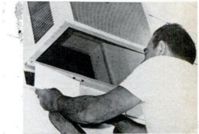
Asbestos shingles are then notched, cut and reinstalled. All ladder work is now completed.
