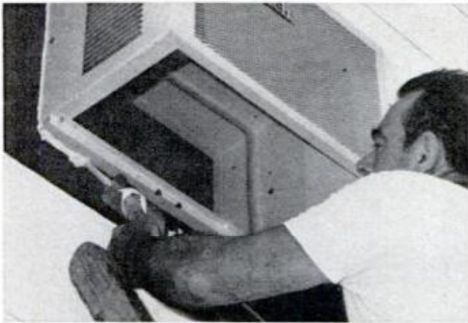
Next, air conditioner shell (exterior housing) is installed, 15-lb. felt is applied and joints are caulked.
