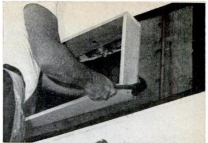
Frame is made on the ground (see drawing below for details), then set flush with sheathing at opening.
