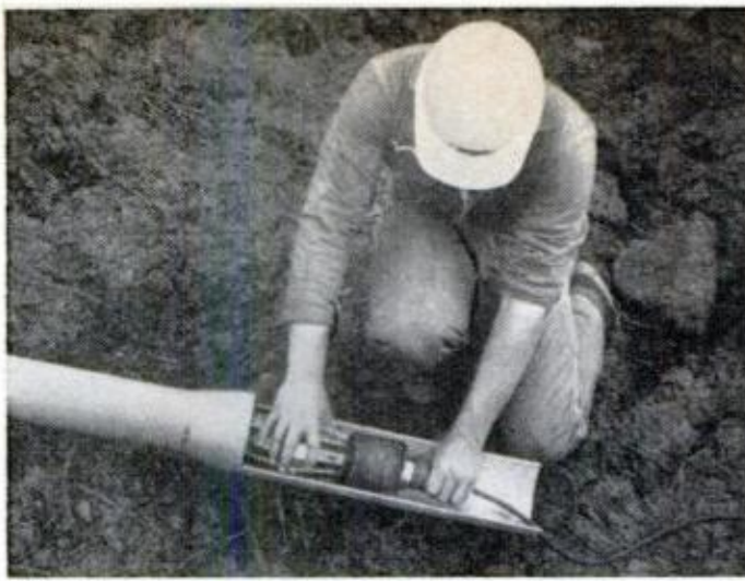
An electronic "pig," shown being introduced into a pipe, detects flaws as it moves along.
