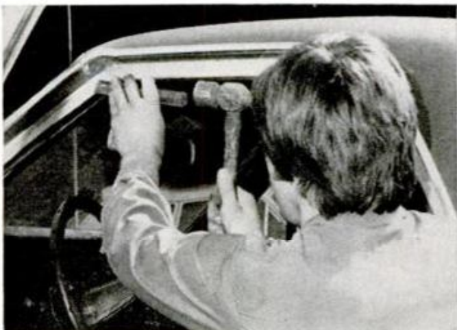
Solder lumps and high spots can be chipped off with a hammer and chisel. Take care not to nick surfaces.
