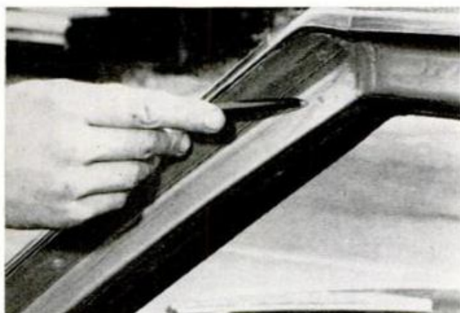
Small construction imperfections such as solder lumps can be the cause of annoying noise around windows.
