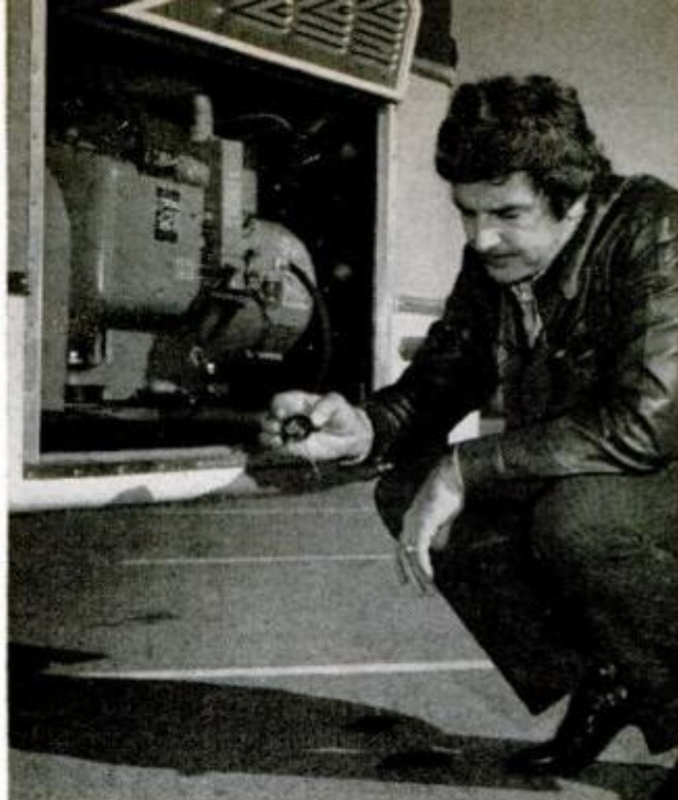
GENERATOR is also powered with an engine needing a daily maintenance exam. Leonard recommends an oil-level check as part of rig's regular "preflight"
