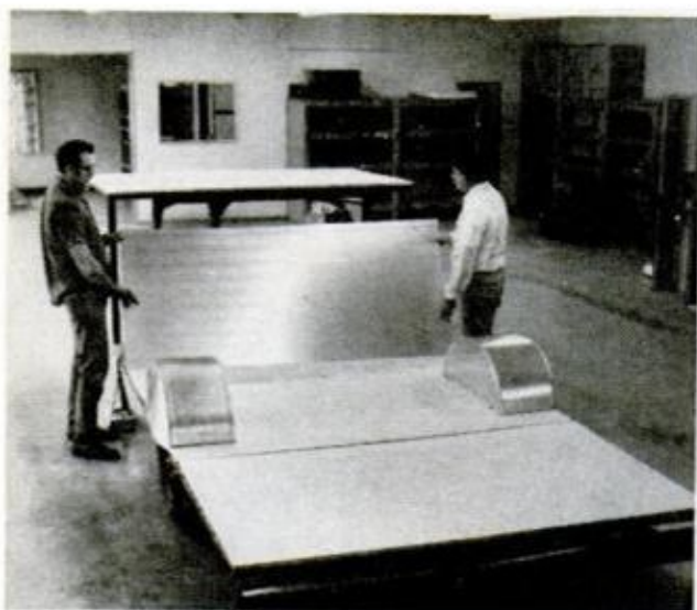
WHEEL WELLS can be farmed out to local sheet-metal shop. When they're installed, flooring can commence
