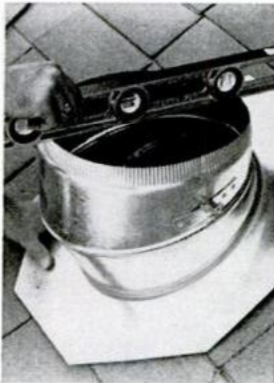
6. WHEN LOOSE, grip top section and turn sufficiently to make the top of the base level
