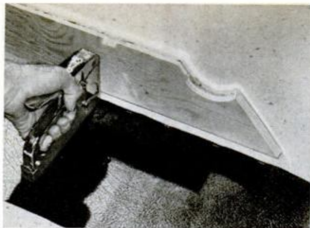
FABRIC-BACKED VINYL is stapled to underside of rails with \frac{3}{16} -in. staples spaced about 1 in. apart
