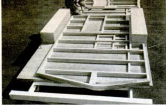
WALLS ARE ASSEMBLED on the trailer floor. It is a must that all studs be exactly the same length
