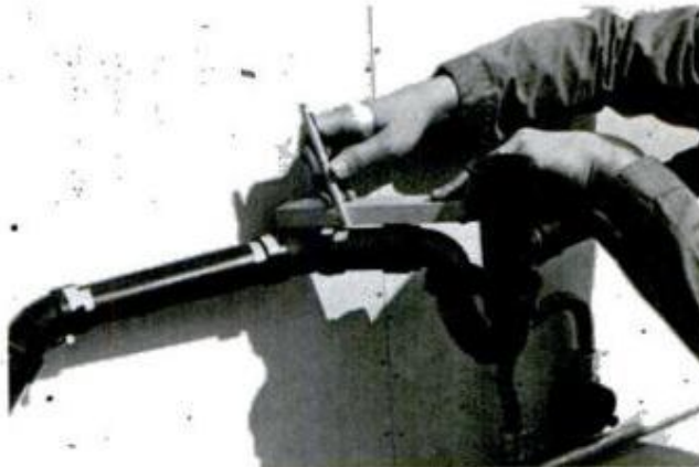
PLASTIC-PIPE DRAIN FITTINGS are taped and a line is drawn to locate relative position of the fittings
