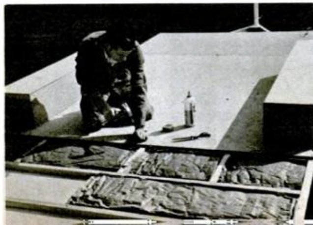
NAIL 3/8-IN. PLYWOOD FLOORING to framework after coating latter liberally with waterproof glue
