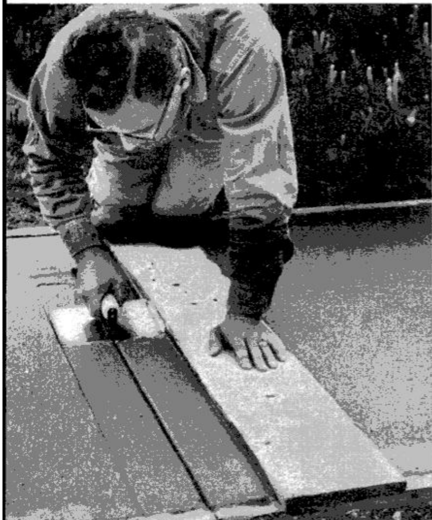
FALSE 'EXPANSION' JOINT is made after slab is troweled
