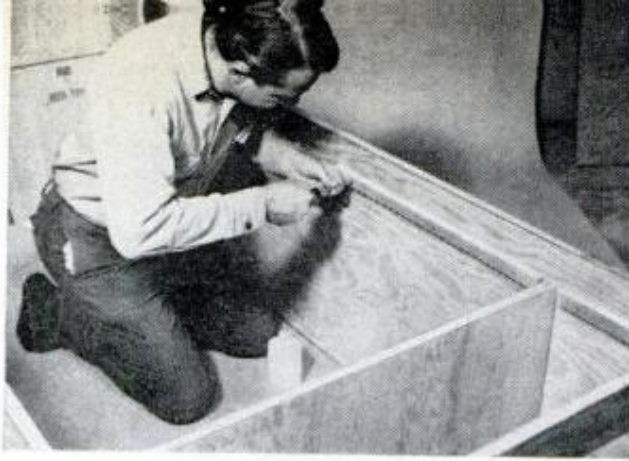
CLEATS SUPPORT PLYWOOD TOP where the mattress rests. They're glued and screwed 3 inches from top
