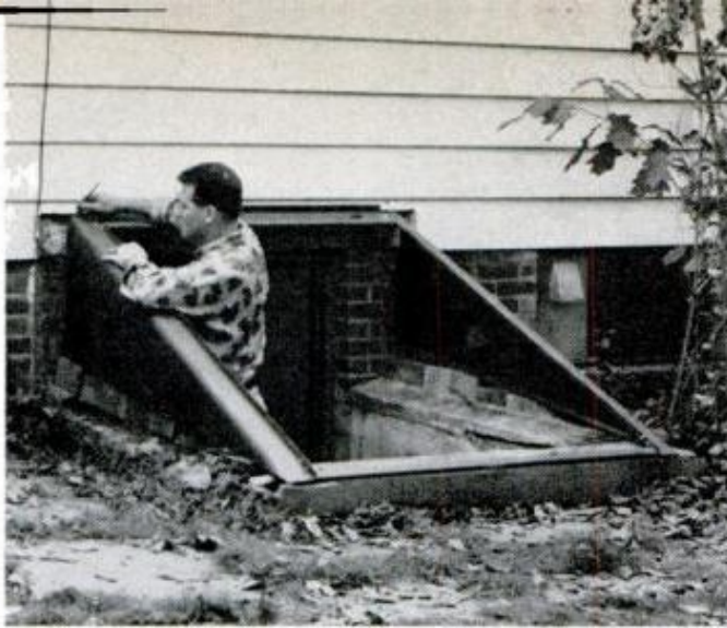
DOOR FRAME is placed in its installation position and siding is marked along top to determine where to cut it
