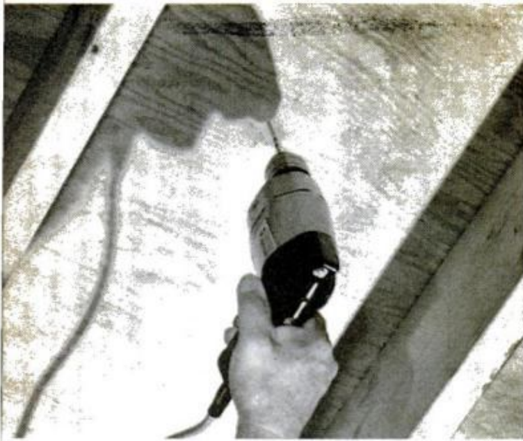
1. AFTER PLOTTING POSITION of fan on roof, drill guide hole from attic to center fan between rafters
