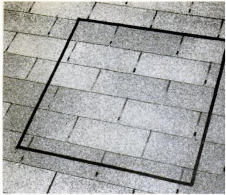
2. USE HOLE IN ROOF as reference point and draw a 27 \frac{3}{8} -in.-square outline on shingles with crayon
