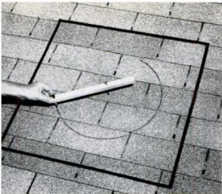
3. MAKE WOOD COMPASS and, using hole in roof as a pivot point, scribe a 17 \frac{3}{8} -in. circle on the shingles
