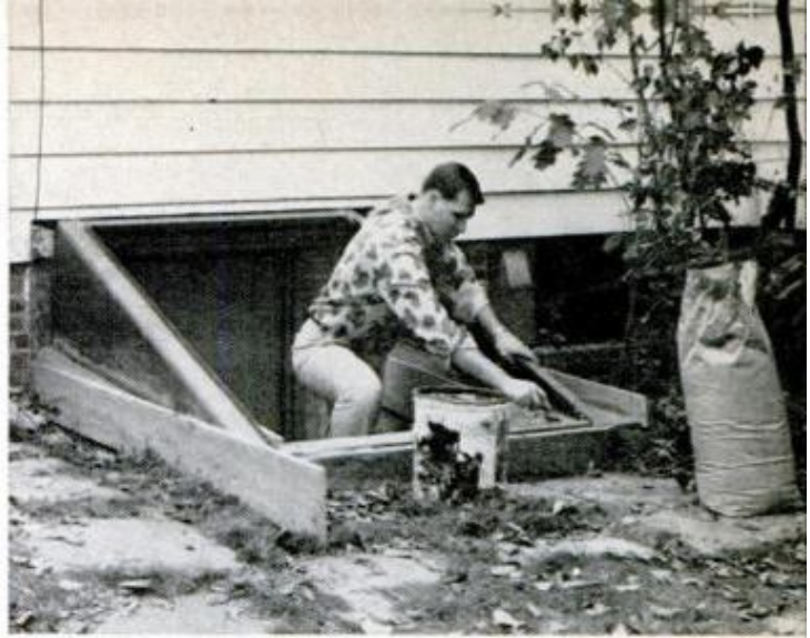
ENTRY IS POSITIONED , fastened to new foundation; joint dressed with mortar where needed
