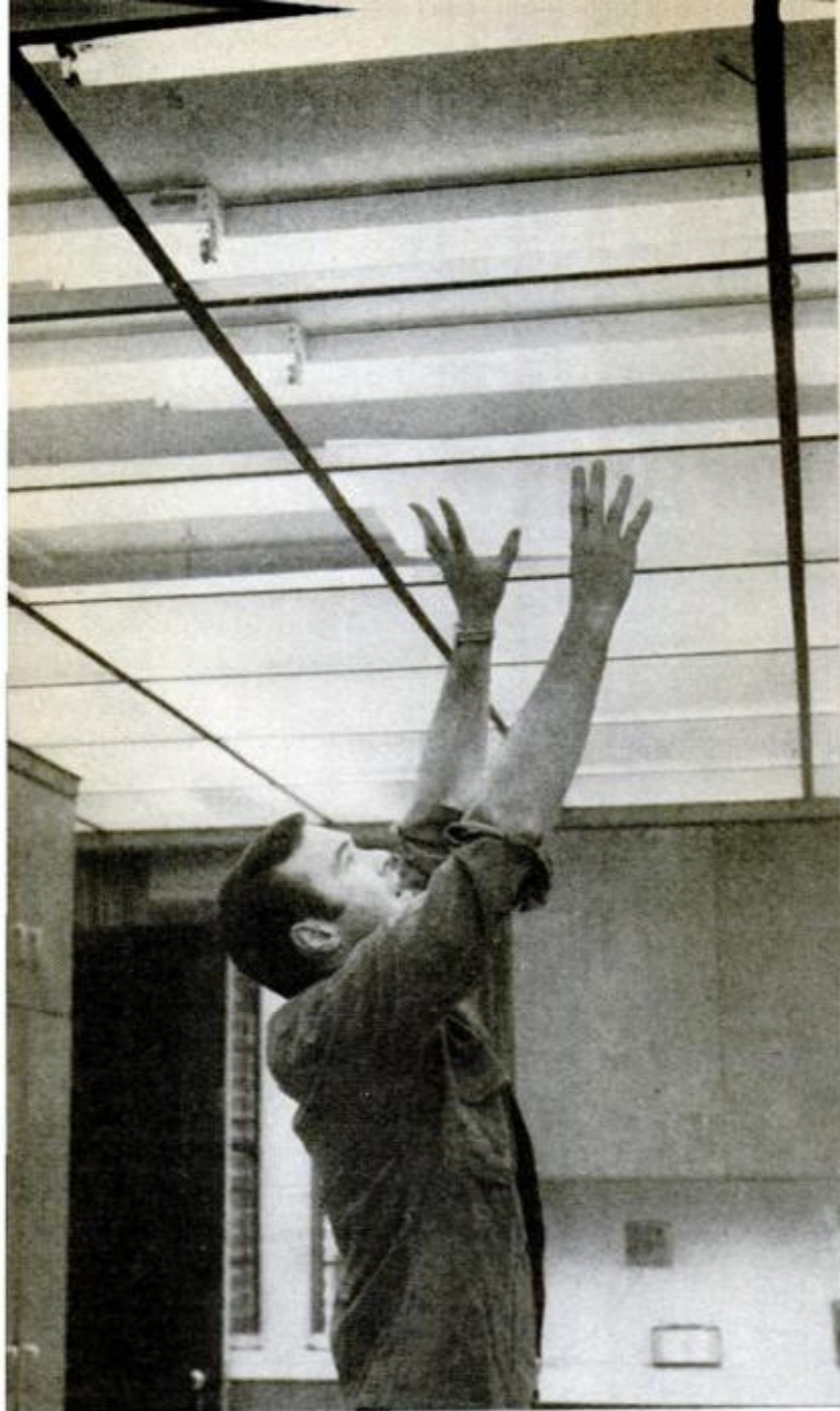
WITH GRID UP , the translucent panels are simply slid into place. Border tiles are the last to be cut and placed
