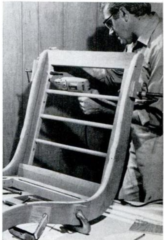
FOR ACCURACY , holes for screws are drilled on the spot with the members clamped in their final position
