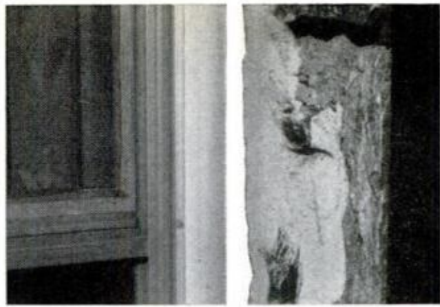
POOR CAULKING leaves end grain exposed. Moisture then creeps in between casing and masonry wall
