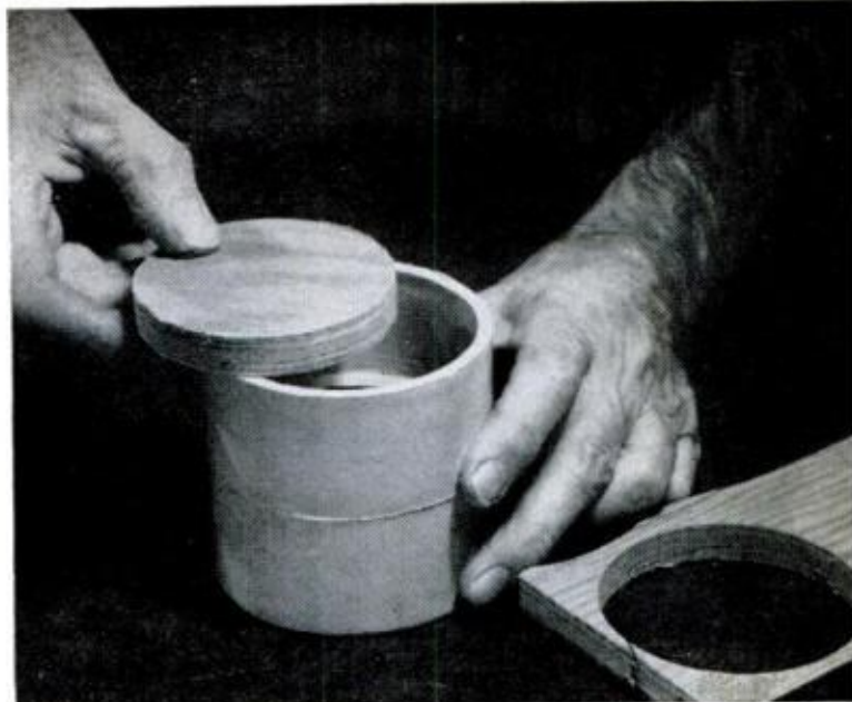
TO PREVENT WALLS from being crushed, simply cut a plug from \frac{3}{4} -in. plywood to fit the pipe's i.d.
