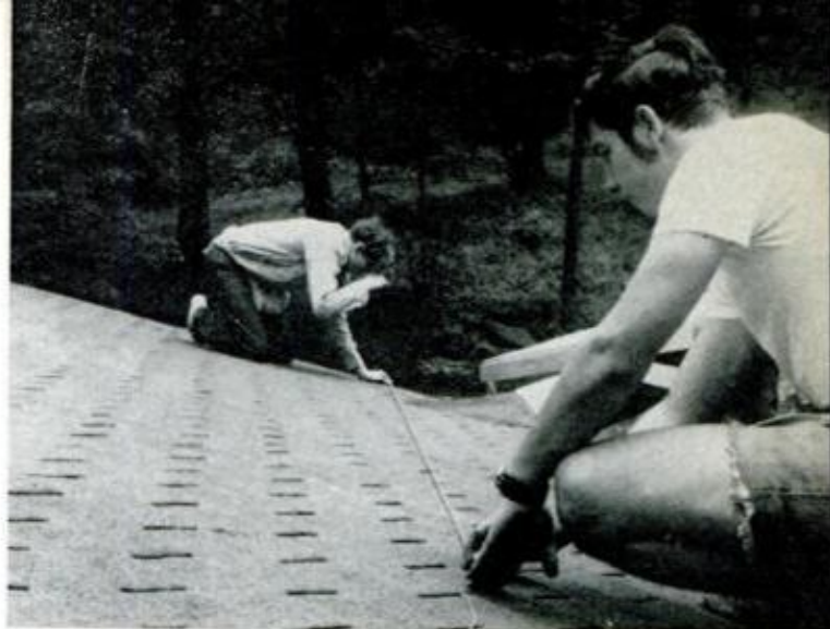
JUNCTION LINE OF ROOFS is obtained by stretching mason line from peak point to the point at edge of old roof where end of the last new truss meets it
