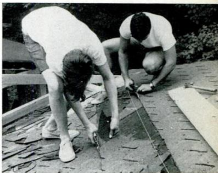
STRIP OF SHINGLES 18 in. wide is removed, mostly inside the mason line, to provide a good, firm seat for the 2x12 plates that will be laid flat against the old roof and firmly spiked into truss rafters
