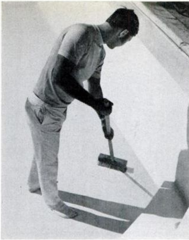
IF CRACKS ARE EVIDENT in a concrete pool, first drain the pool, then patch and thoroughly clean it
