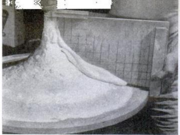
FINAL SHAPE is made by screeding patching plaster with special plywood screed built as shown in drawing
