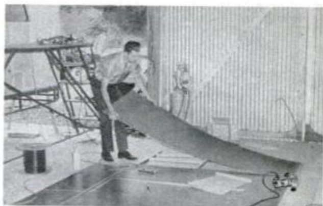
PREFINISHED PANELING is stapled to sidewall frames after glue bead has been applied to studs
