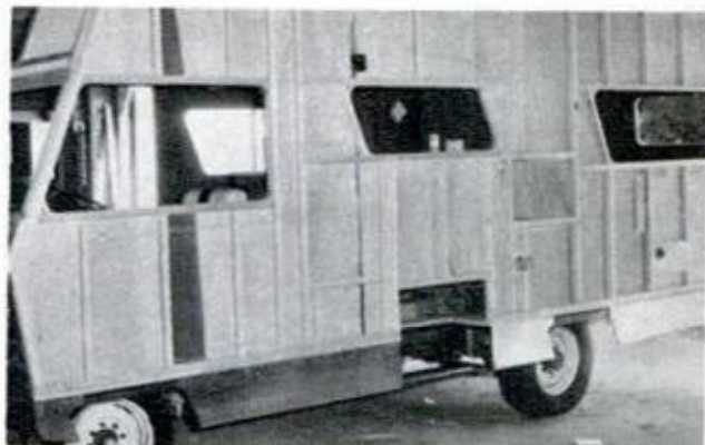
LEFT SIDE WALL ready for aluminum exterior "skin." Styrofoam (1 in. thick) fits snugly between all studs
