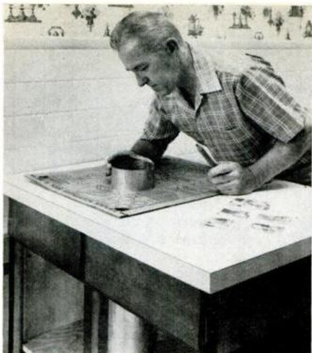
3. REPOSITION TEMPLATE over cutout and use it to locate vent-pipe hole. Here pipe runs through floor
