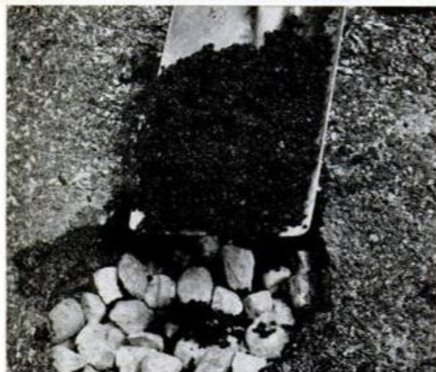
EXAMINE DRIVEWAY , then fill large holes with stone and complete patching with a suitable patching mix
