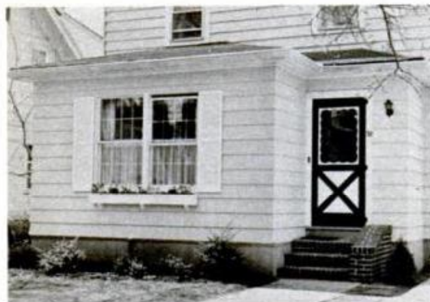
AFTER: Double window meets FHA minimum requirements; rebuilt room functions for everyday living
