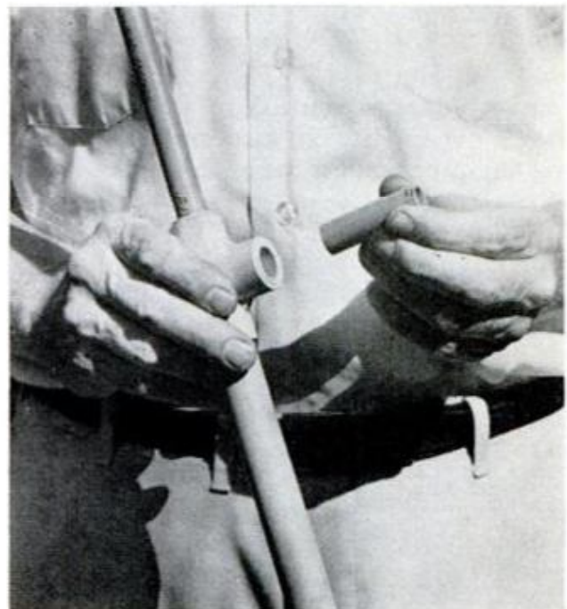
WITHIN A MINUTE of starting to dope the joint, insert the pipe into the fitting with a slight turn
