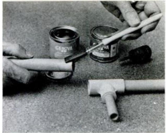
BRUSH SOLVENT No. 1, then solvent No. 2 on the end of the pipe and on the inside of the fitting
