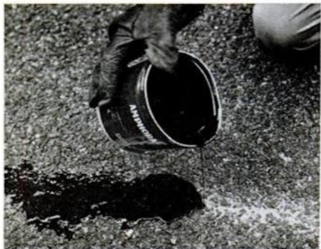
SMALL CRACKS and holes can be treated with a crack filler. Let the cracks cure for at least one week
