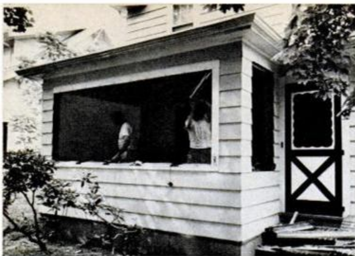
WITH A FRIEND HELPING , author knocked out windows in one day and had the room closed in by sundown. Opening was stripped down to the wall studs before any rebuilding was started. For safety, keep the work area free of debris
