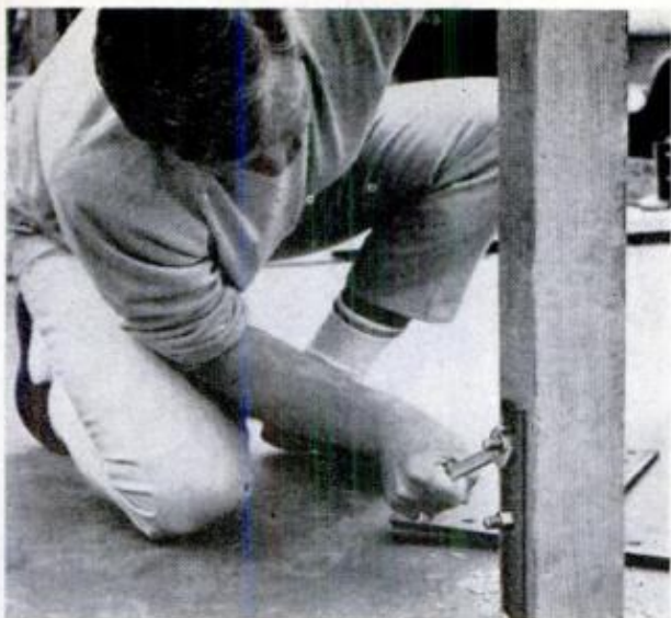
CORNER POST is bolted to bracket planted in concrete. To avoid rust stains, use galvanized hardware
