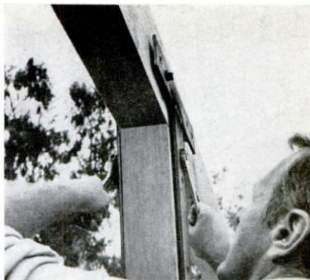
T-SHAPED BRACKET used to fasten beam to post is fast method, provides rigid, strong construction
