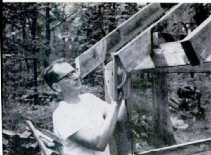
AFTER PLACING RAFTERS , plumb the ends with level, then cut them off in place with portable circular saw. If using old timbers, check for nails before cutting
