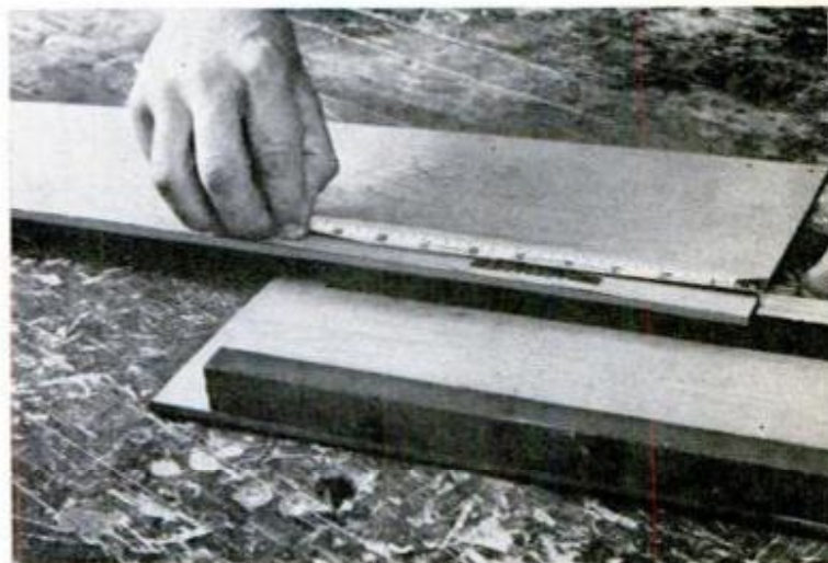
WALL HANGERS are located equidistant from both ends and fastened in place. The panel edges are finished with a single coat of flat black enamel
