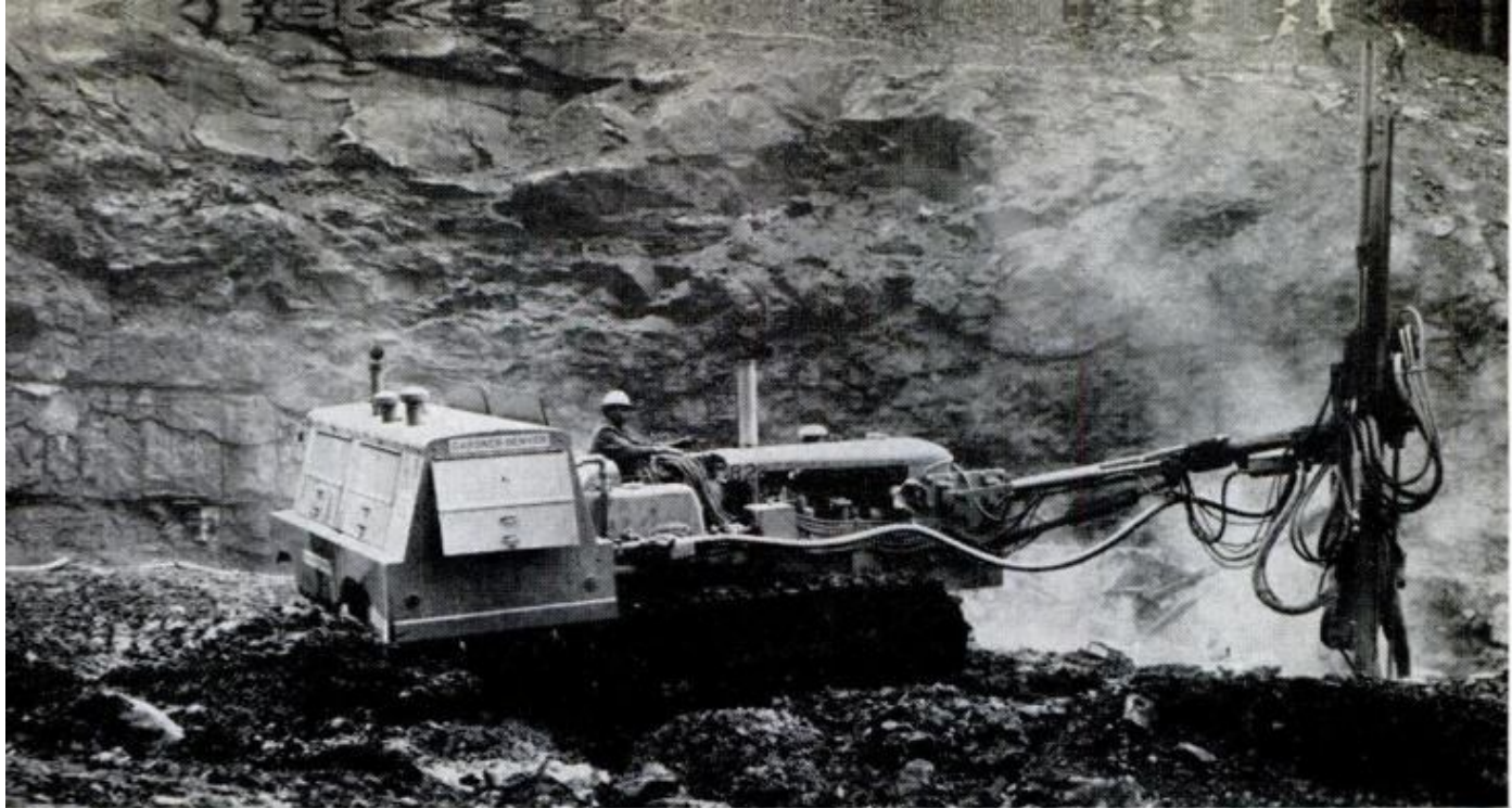
BIGGEST PIECE OF EQUIPMENT is new 40-ton crawler tractor with Gardner-Denver Rota-Screw portable compressor mounted on the rear, boom and drills mounted in front. Drilling is done from the driver's seat
