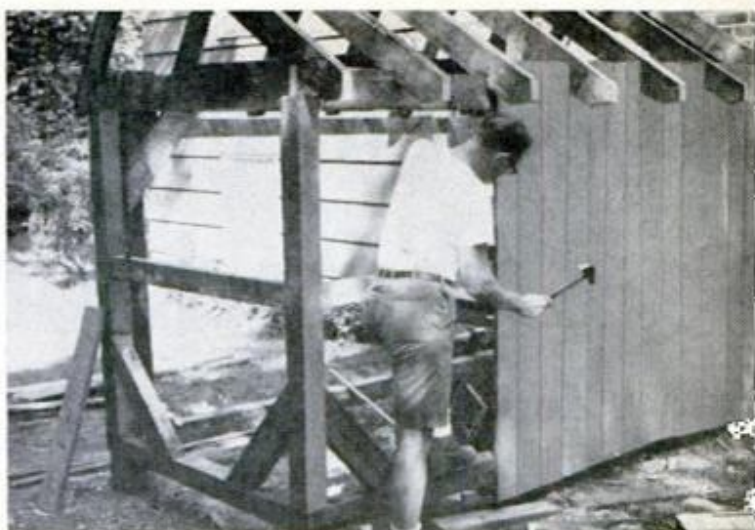
SHED IS SKINNED with one-by sheathing applied vertically. Notice horizontal members placed between uprights to provide midpoint nailing and rigidity
