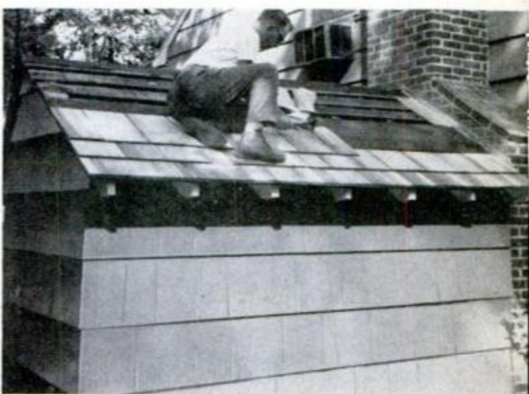
RESAWN CEDAR SHINGLES used on roof were applied with 4-penny galvanized shingle nails (two per shingle). For long life, preservative was applied next
