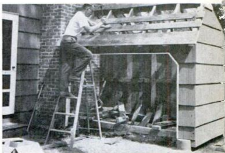
WIDE ONE-BY STOCK was used for furring; boards are spaced about 12-in on center so that shingles can be applied with 8 in. exposed to the weather
