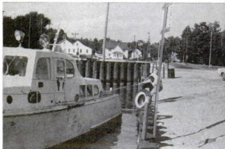
NO DOCK, NO FINGER PIER, no ladder and inadequate fendering—basically a miserable arrangement!
