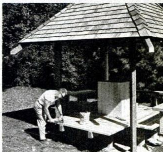
PIER-SUPPORTED BEAMS are decked with 2x4s placed flat and 1/4 in. apart. Use 12d nails
