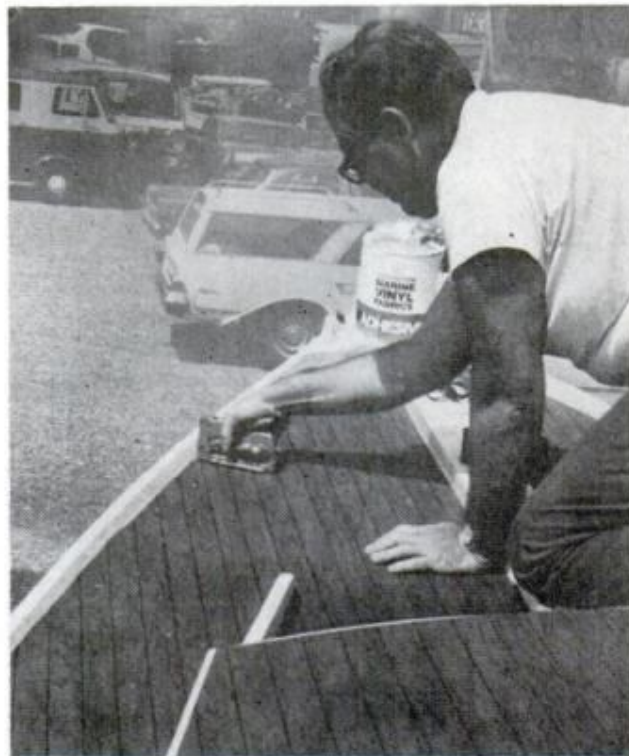
NEXT-TO-LAST STEP is to fasten edges with staples to hold vinyl until glue sets. By working carefully, deck-seam lines were matched for best effect
