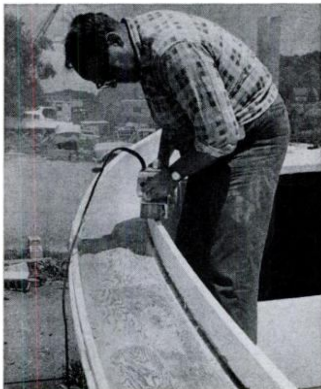
HEAVY-DUTY BELT SANDER is used to rough plywood undersurface before installing the vinyl. Plywood was wiped with acetone to clean it and dry out moisture
