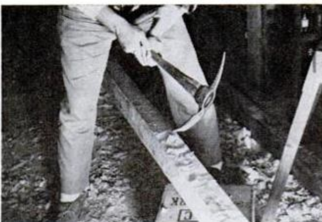
EASIEST METHOD of adzing is to straddle raised beam. Use workstop or clamps to prevent movement
