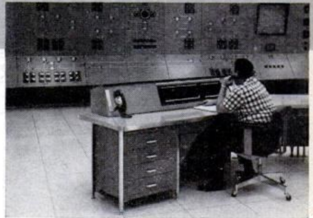
CONTROL ROOM at Levis substation. Lines also serve as a telecommunication system between substations
