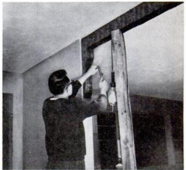
POST SUPPORTING BEAM stays put until all bolts are turned home. Knee is fastened to wall next
