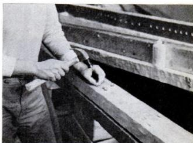
COATED WITH GLUE , the plugs are then driven into enlarged nail holes before adzing operation begins
