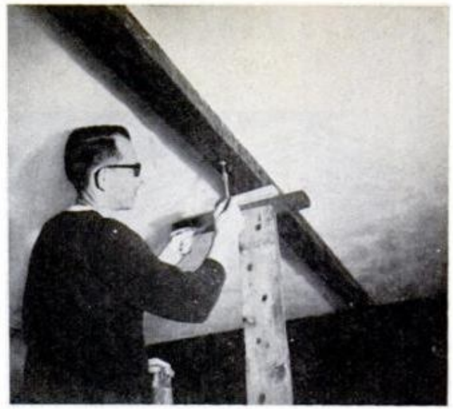
PREDRILLED BEAM is positioned over chalkline, held fast by T-support wedged with shims, then bolted
