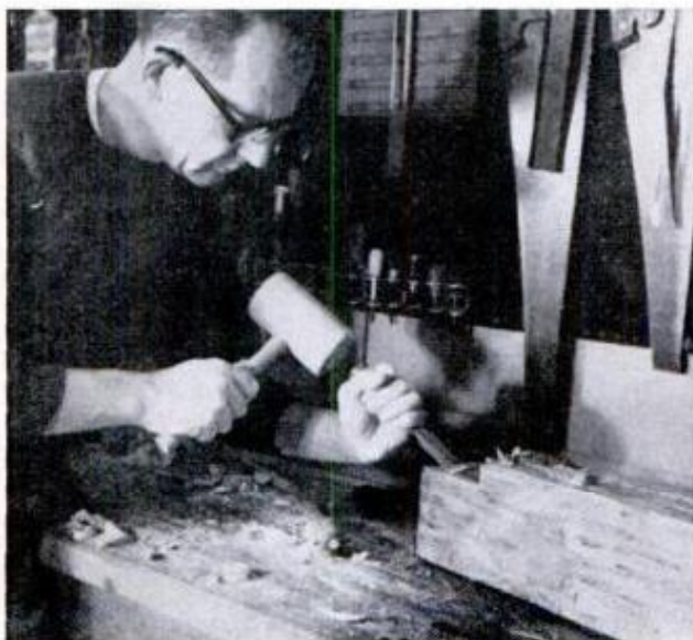
BEAM END is chiseled out to receive wall-knee support. Kerfs made with a power saw speed this step
