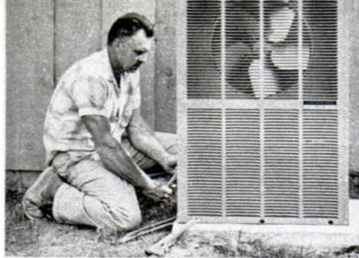
CENTRAL AIRCONDITIONING compressor was installed outdoors. Evaporator is in furnace plenum
