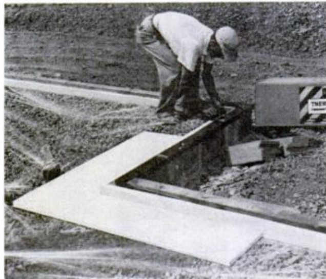
SLAB HOUSE construction calls for rigid insulation placed around perimeter. Notice vapor barrier
