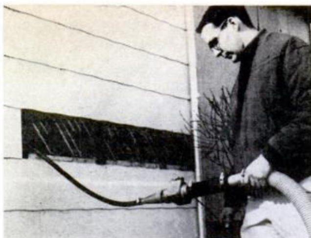
BLOWN-IN installation requires special knowledge and equipment, is a chore best left to the pros
