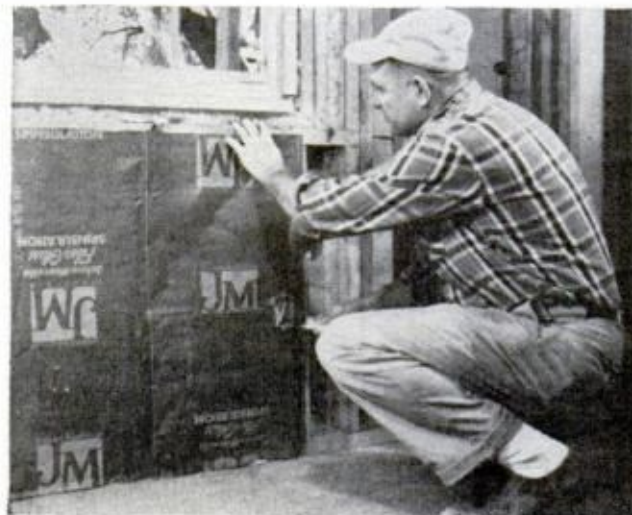
STAPLING FLANGES are lapped over studs, provide vapor barrier. Notice loose insulation around jamb
