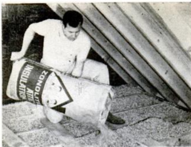
VERMICULITE ATTIC INSULATION used to beef up inadequate insulation is poured between joists
