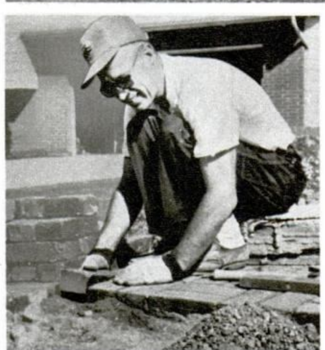
SPACE THE BRICKS \frac{1}{8} to \frac{1}{4} in. apart so white sand later can be swept into the cracks even with top
