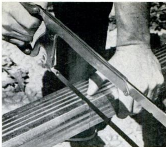
DOWNSPOUTS AND GUTTER sections are cut with a 32-point hacksaw. Support the section solidly and keep the blade flat as possible to avoid pinching
