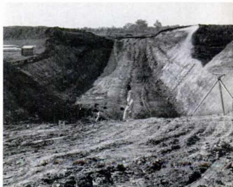
MOUNTAINS of earth must be moved to carve new track. Here engineers check Talladega infield access
