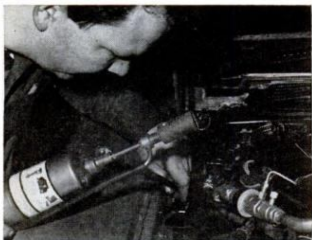
PROPANE TORCH , with an adapter and sniffer tube attached, is used to check for leaks in system. Leaking refrigerant will change color of the flame
