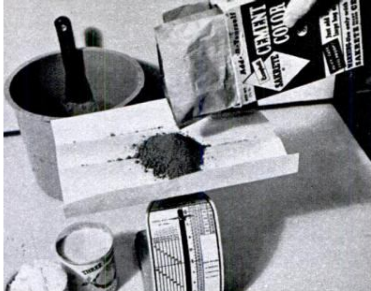
KEY TO COLORING CONCRETE is to use weighing method of mixing, not coloring by volume. This is true of both dust-on and integral-mixing techniques
