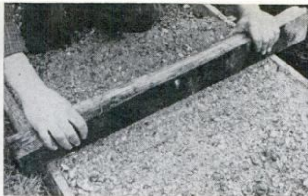
POUR A BED OF CONCRETE and beat the mix down with a length of lumber. Make sure the form is level
