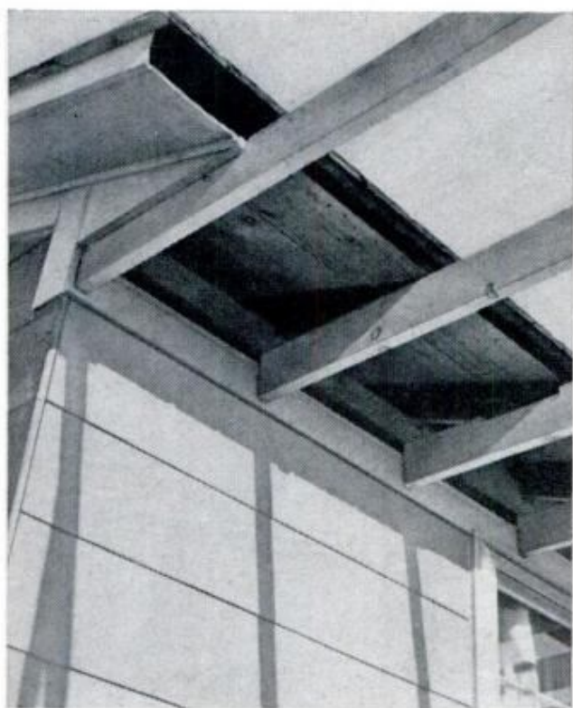
CEILING JOISTS are toenailed to a 2x6 nailer which is first nailed to the house at ceiling height
