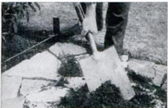
SPREAD FINE SOIL over the completed walkway. It often is advisable to sift all the topsoil first
