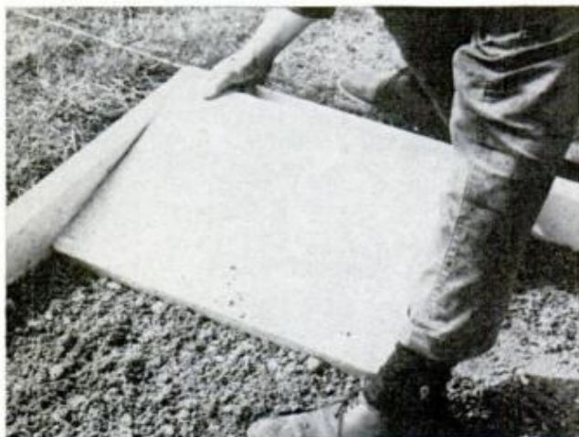
CAREFULLY POSITION SLABS over loose soil. It's a worthwhile idea to first chart your layout of slabs
