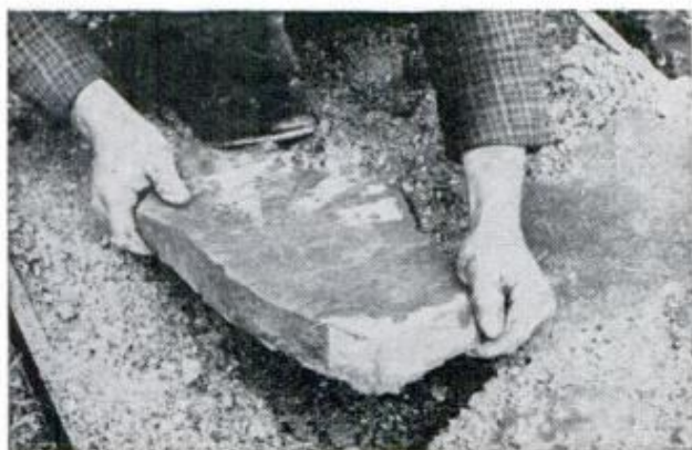
WHILE CONCRETE IS STILL SETTING , scoop out portions and inlay stones, slabs or other material
