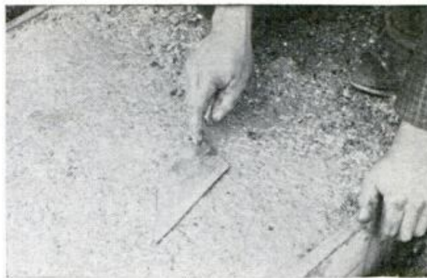
USE A TROWEL in pounding fashion to bring fuzzy finish to surface. Smooth walks can be dangerous
