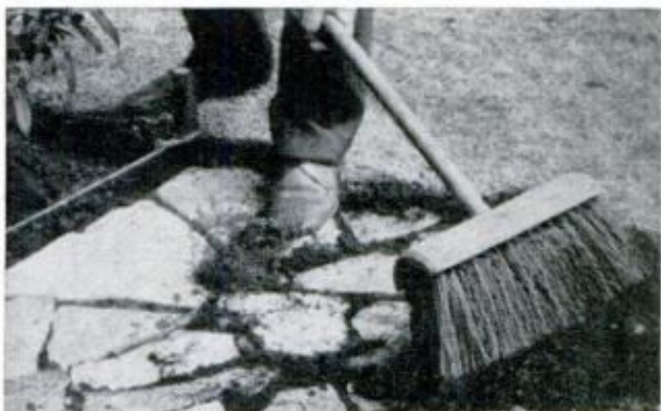
BRUSH THE SOIL into all the cracks and crevices at butt joints to produce a well-defined walkway
