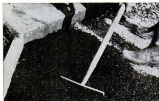
RAKE OUT ASPHALT AT ONCE. Heating the head of the rake over a low flame makes raking task easier
