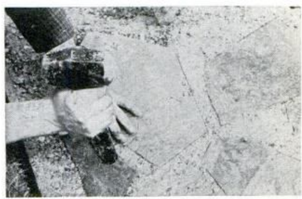
TAMP DOWN until level. The cement will be forced up between the joints to be flush with the surface
