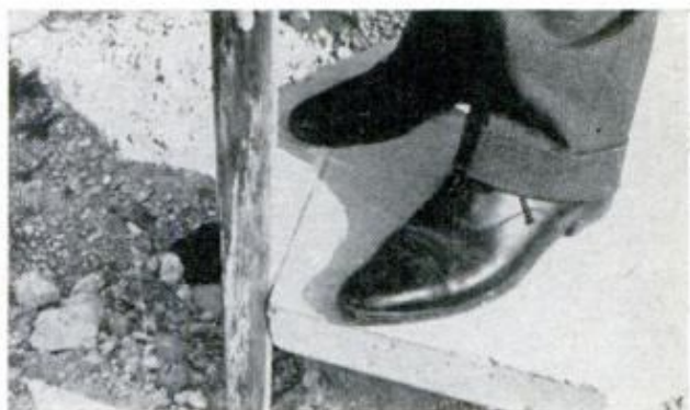
USE A MASONRY SAW to cut between the drawn lines, applying water liberally to lubricate the saw
