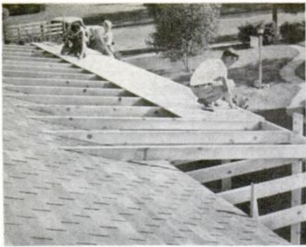
TAPERED ENDS OF RAFTERS rest on house roof to which they're nailed 24 in. o.c. Plywood covers rafters
