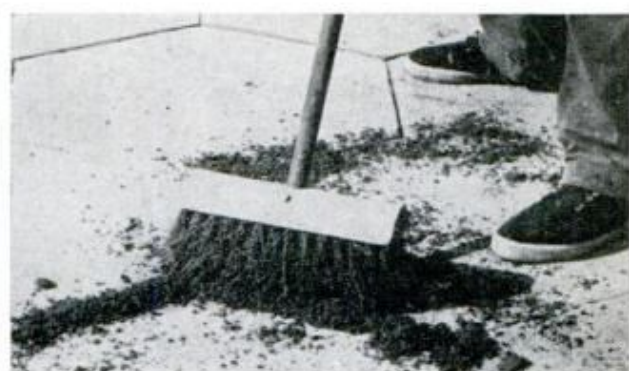
FINE, SIFTED SAND is then brushed into all cracks until every joint in the walk is completely filled
