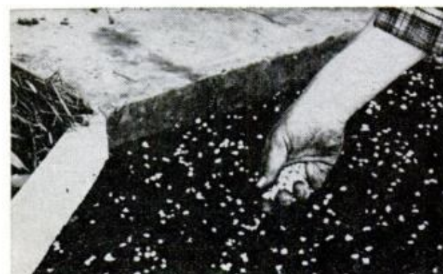
A SPRINKLING OF COLORED CHIPS will break the solid color and improve appearance. Then roll path
