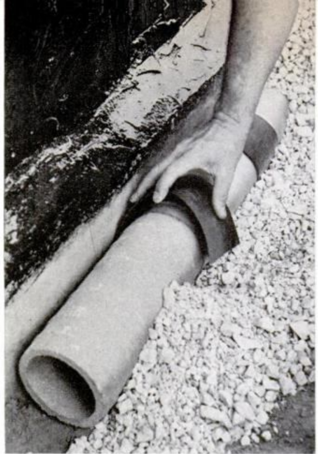
IN WET AREAS , foundation drain tiles can make all the difference between a dry or flooded basement
