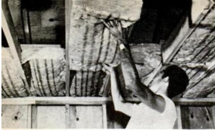
EXTRA-THICK INSULATION , like these 6-in. batts between ceiling joists, indicates good construction
