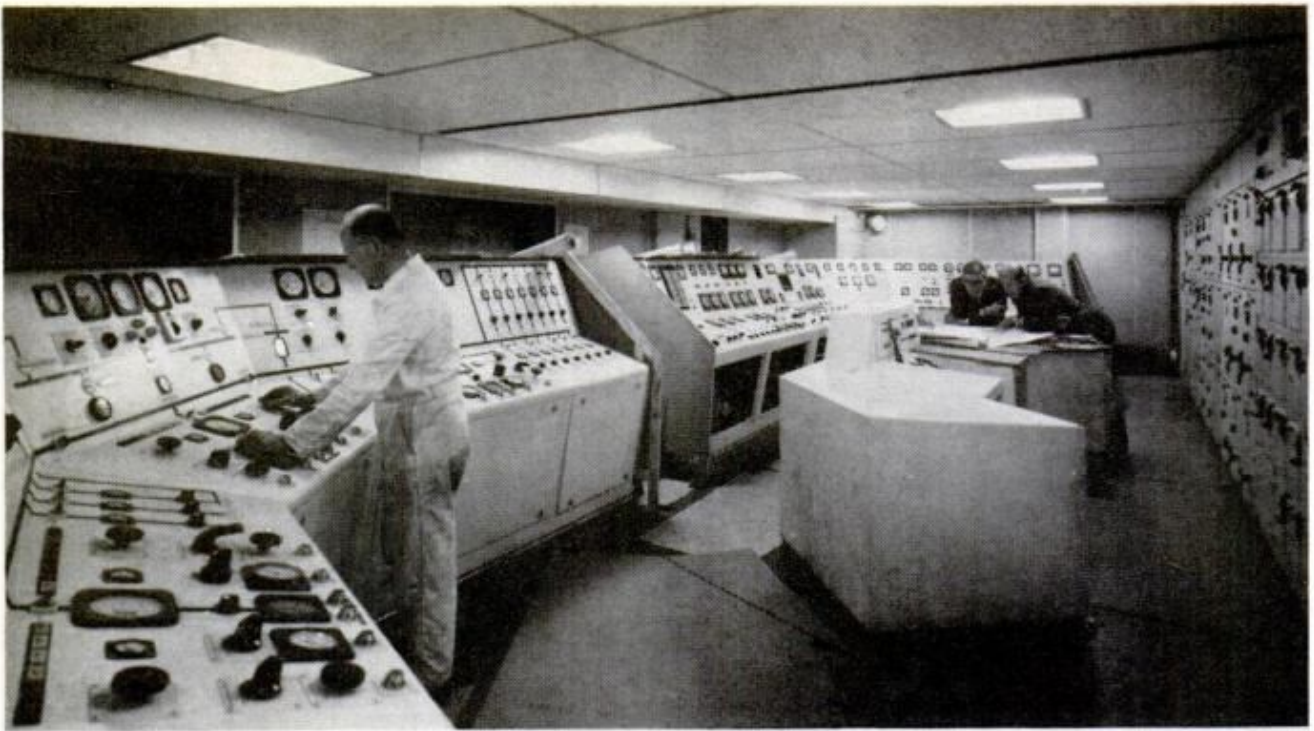
MAIN CONTROL ROOM features pushbutton consoles that direct electrical distribution, power supply, air conditioning, stabilizers and other major mechanical operations
