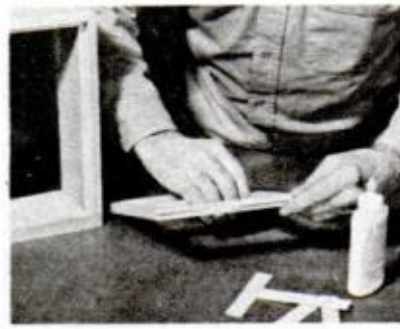
AFTER GLUING butt corners of door frame, \frac{1}{8} -in. splines are inserted, glued and trimmed flush
