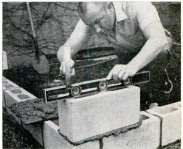
CORNER BLOCKS are laid to interlock. These govern position of all other blocks, so level them both ways
