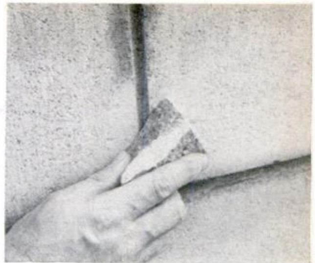
MORTAR DEPOSITS on face of wall can be rubbed away with a piece of broken block after hardening
