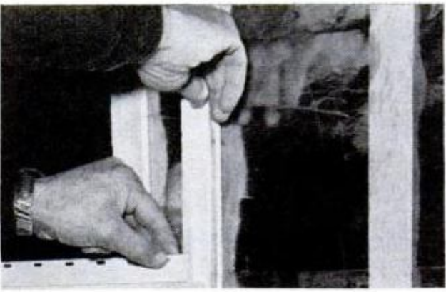
JOINTS IN SIDING should always be reinforced with backer. This makes entire panel more rigid
