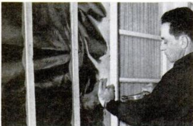
INSTALL TRIM PIECES around doors and windows and in corners before you begin nailing siding
