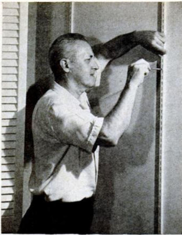
SLOTTED STANDARDS , 5 ft. long, are screwed to the studs in the back wall of the closet for solid support
