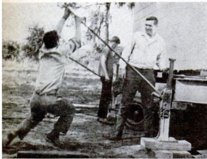
AT THE NEW SITE , house is jacked up so wheels can be removed from underneath. Temporary blocking will be built up around jacks to take main weight
