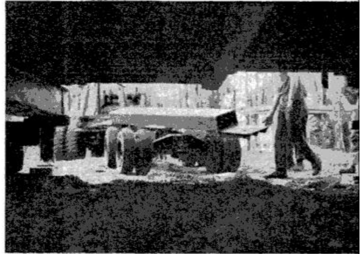
WITH HOUSE BLOCKED UP , wheels are pulled out. Foundation walls will then be built up to fill the gap and the house will be jacked gently onto them
