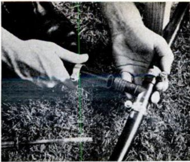
LATERAL LINES are attached by means of a T-joint spliced into main line. System shown here is Buckner's
