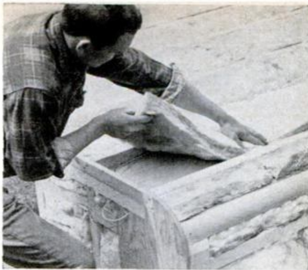
FIBERGLASS INSULATION is well worth the slight added expense. Note that the front 2x2 has been rounded off to conform to shape of plywood gusset
