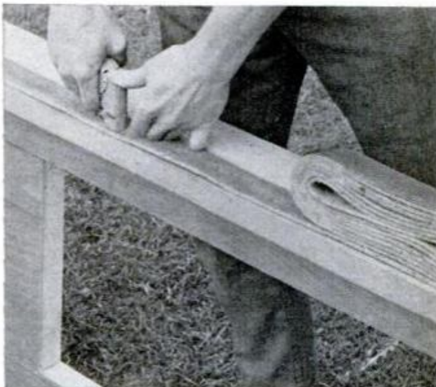
WEATHER SEAL between the shell and the truck box is just weatherstripping stapled in place. The extender should have same seal, both top and bottom
