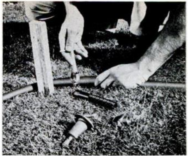
SPECIAL TOOL cuts hole in pipe at sprinkler head location. Riser is then attached with a saddle clamp
