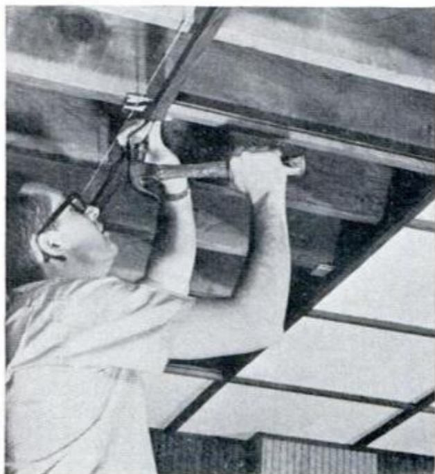
MAIN RUNNERS ARE NAILED directly to joists. Use the cross runners to help determine the exact spacing
