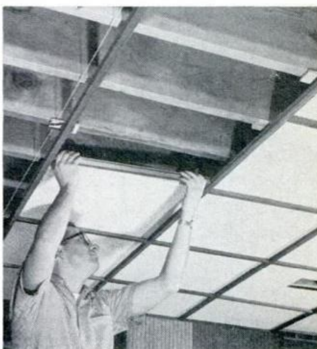
SLIDE IN DECORATIVE PANELS , either 2x2 or 2x4-ft., then frame them by sliding in mitered cross runners
