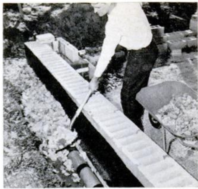
CLAY FIELD TILE laid in ditch along footing of wall and covered with gravel, drains seepage from bank
