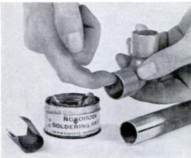
CLEAN THE OXIDE from the tube and the sockets with fine abrasive paper. Then wipe on rosin paste flux
