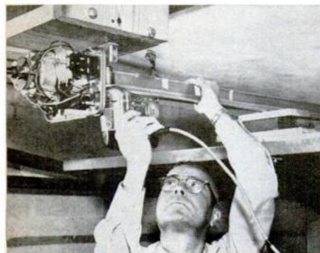
OPEN DOOR supports track when anchoring motor end to bridging, permits working without helper
