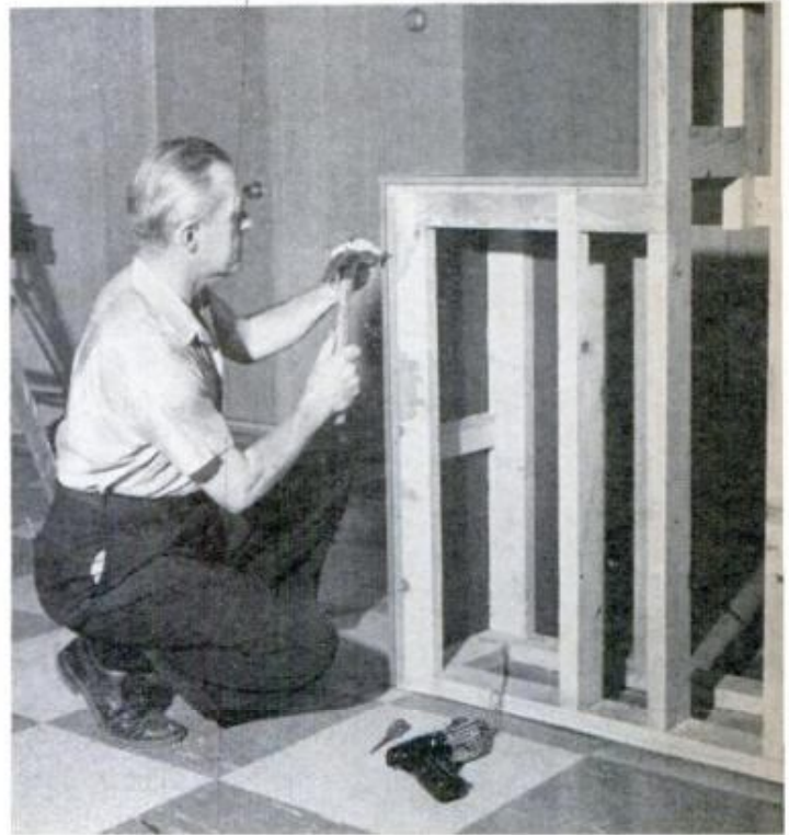
EDGES OF PANELING at corners are concealed by a matching metal molding which is nailed to framing
