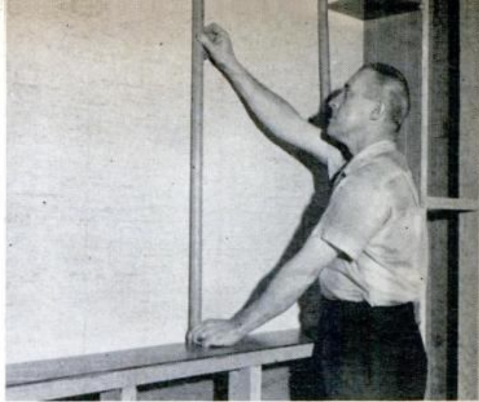
STICKS ARE USED to hold top and bottom panels in place when cementing lining in bookcase recess
