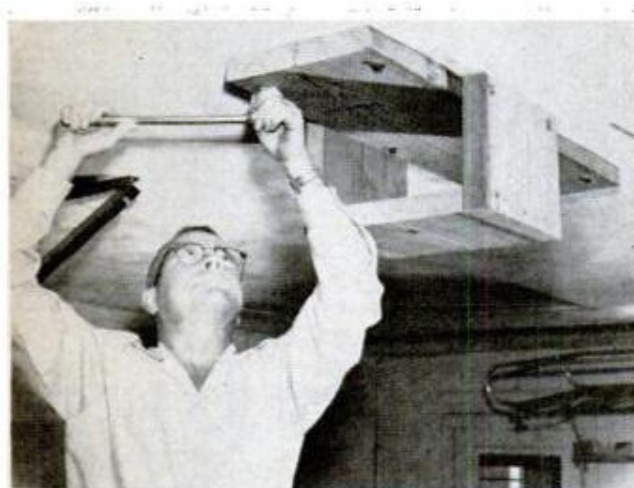
BRIDGING TO SUPPORT MOTOR END of track is long enough to span three joists and bolts to them
