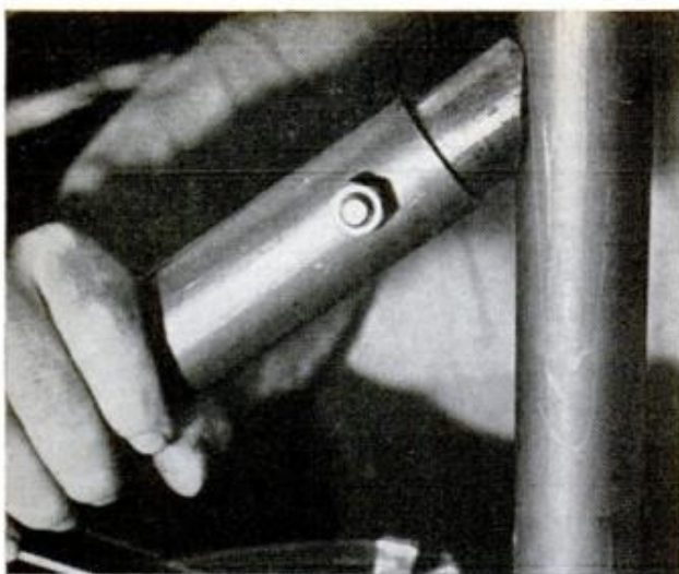
SLEEVE MUST BE ANGLED where it contacts the rollbar to produce a strong, safe joint between the two
