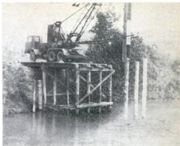
HOMEMADE PILE DRIVER was used to pound logs for bridge into tempestuous river that often overflows
