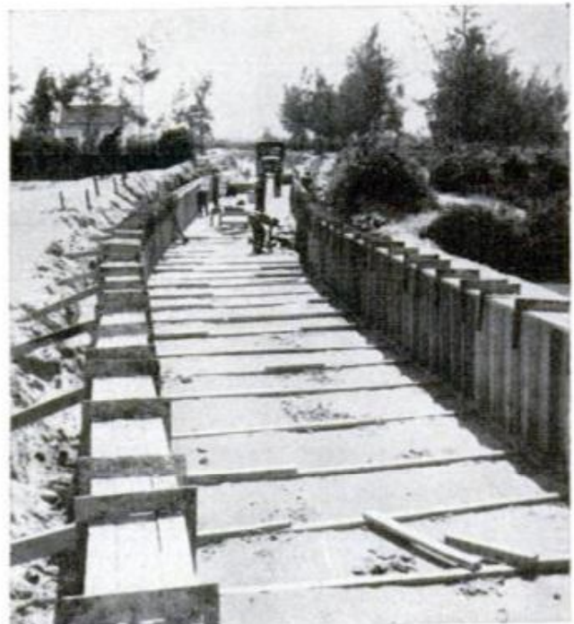
HEAVY RAINS in Vietnam require many drainage culverts to prevent erosion of roads and airstrips
