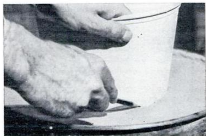
LILY TUB , used as form for lid plug, is first fitted in refractory opening, marked, then cut \frac{3}{8} -in. below this line
