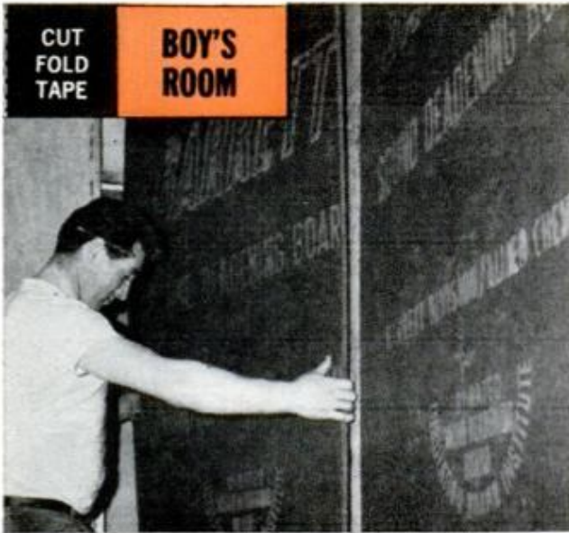
SOUND-DEADENING BOARD is applied to all partition walls. Here it's being fitted between the tracks
