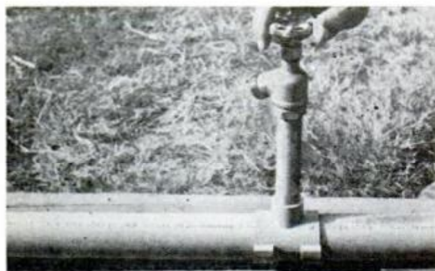
DRAW SLIDE-ON CLAMPS around pipe and insert them in slots on fitting. Finally, thread in nipple
