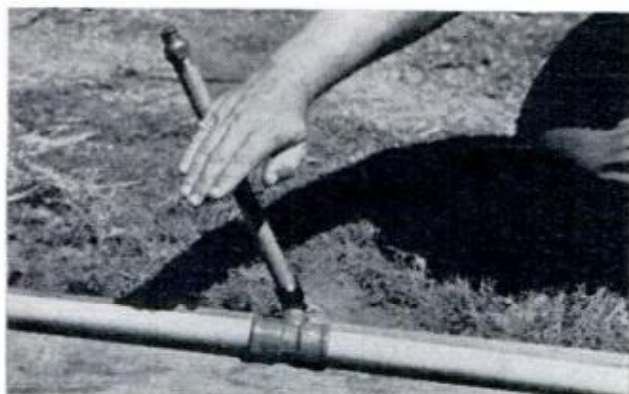
PREVENT DAMAGE TO RISERS by using PVC tee fitted with a plastic street-elbow in center socket
