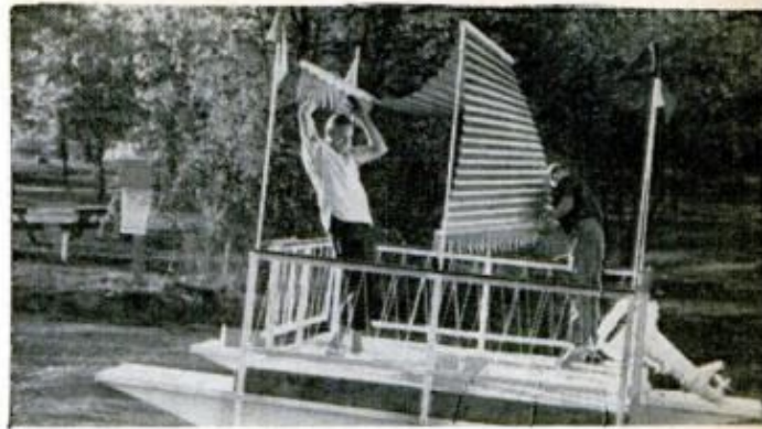
SLIP RIDGEPOLE sockets over center pair of conduit supports before bolting end boards to corner poles
